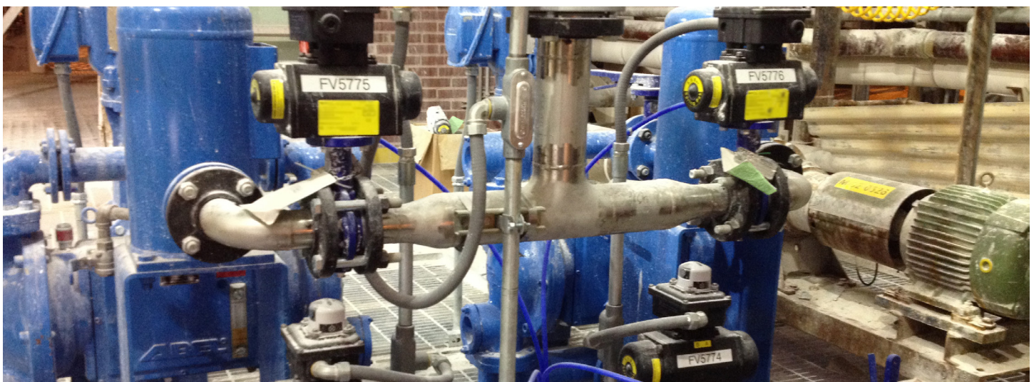
ABEL EM-50 electric diaphragm pumps for filter press feed.
